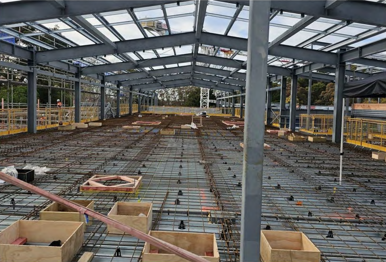
10073 Te Pae Tawhiti Adult Mental Health Facility, Waikato Hospital Level 2 preparation of concrete pour
