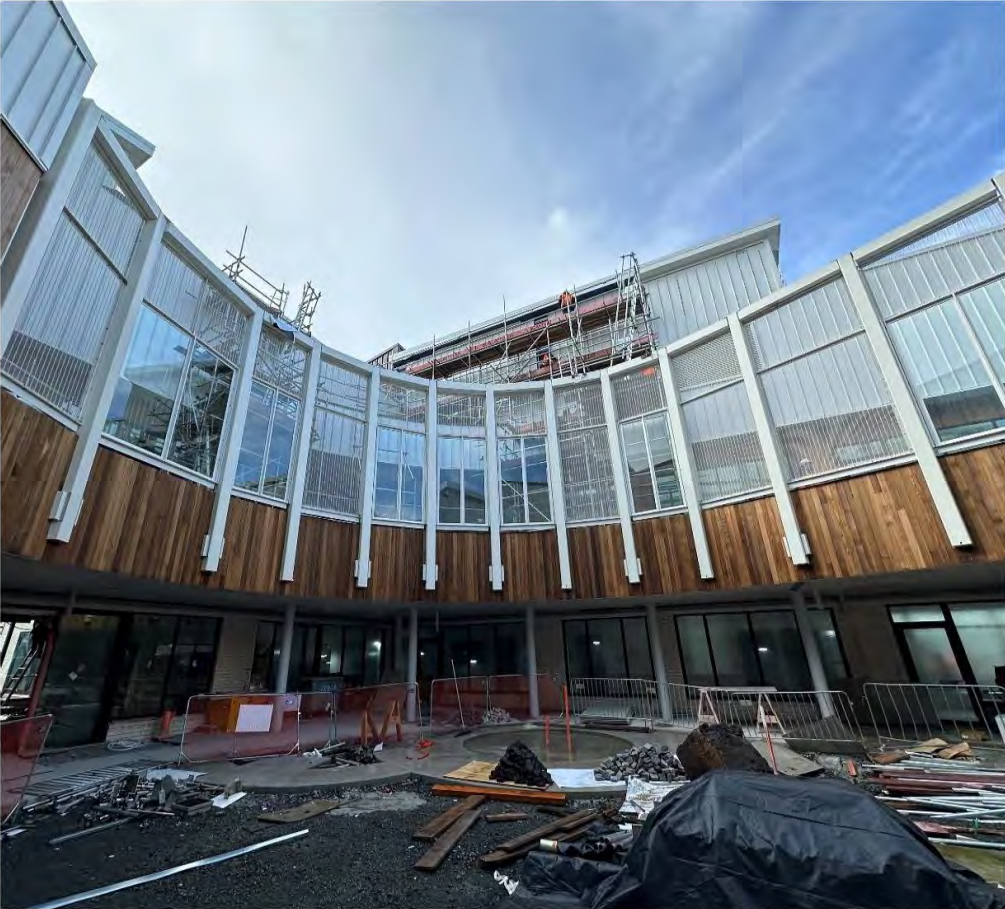
10050 E Tū Wairua Hinengaro - Forensic Psychiatric Services Facilities Replacement, Mason Clinic, Auckland Western courtyard terrace screening
