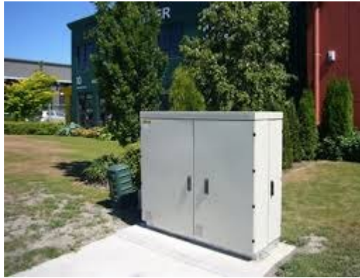
Figure 16 – Externally located outdoor telecoms cabinet on a concrete plinth.
